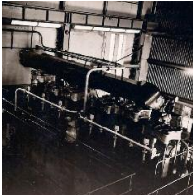
Figure 7 View of top of No 5 set which was installed without covers
