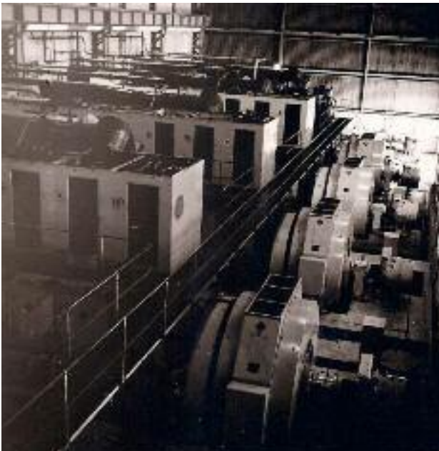
Figure 6 General view of 2, 3, 4 & 5 H&W sets taken from the station crane
