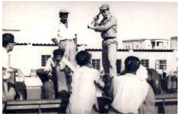
Figure 5 Mike Bradley tightening nuts on main bearings Note use of rope to maintain tension on spanner. The bed plate and crankshaft appear to have been shipped part assembled.
