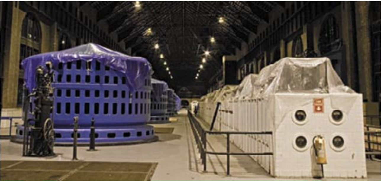
Figure 20 Taraulins cover mothballed generators and electrical equipment - "current" situation in William B Rankine powerhouse
