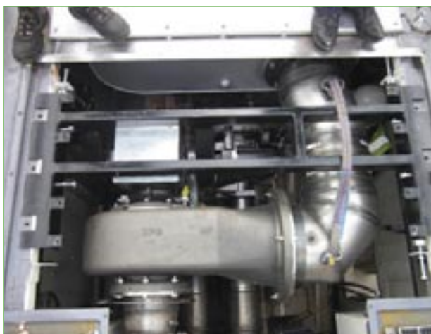
Figure 3: ETC installed in containerised genset
