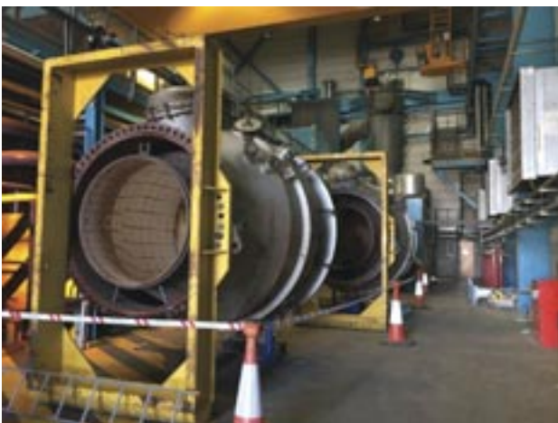
Figure 6: GT Combustion chambers in turbine hall
