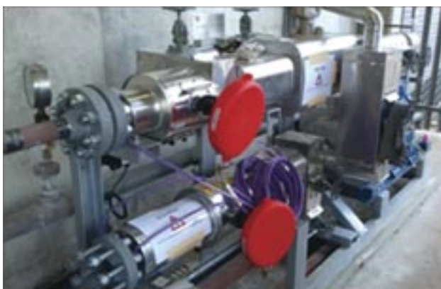
Figure 12: New water recirculation skid for fuel gas preheater
