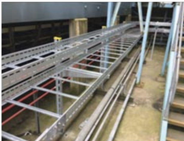
Figure 13: Cable racks for new communication and power cables
