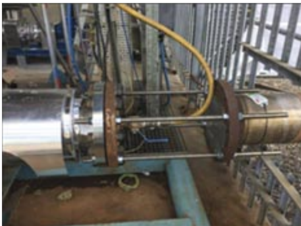
Figure 11: Air-gap in fuel gas supply pipeline during preservation
