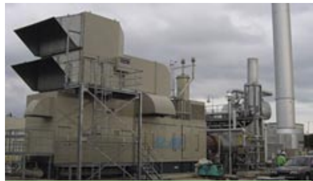
Figure 7: 7MW class gas turbine in Japan operating on vaporized LPG
