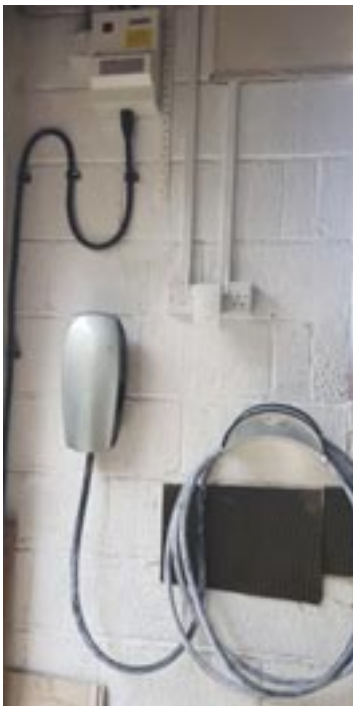
Figure 3: 7kW charger with garage consumer unit and cable reel (plus wifi extender!)
