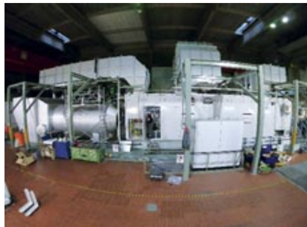
Package installed & awaiting systems checks
