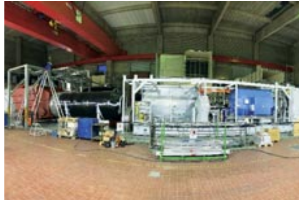
The installed exhaust gas silencer and boiler
