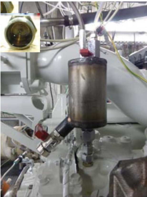
Figure 1: Accumulator and Orifice
