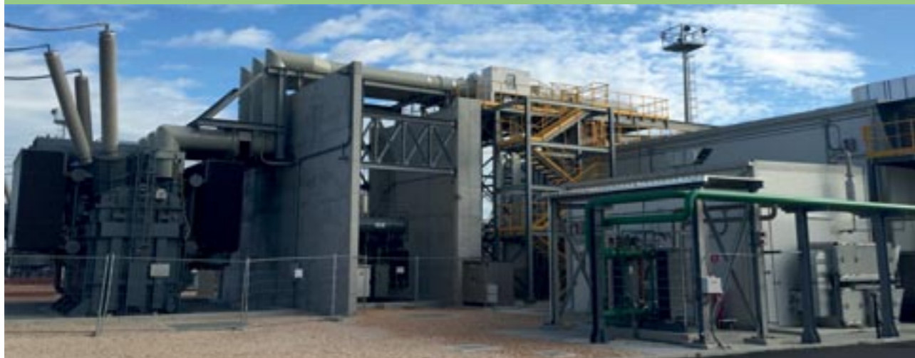
Figure 10 – Site photos - Close view of Synchronous Condenser plant
