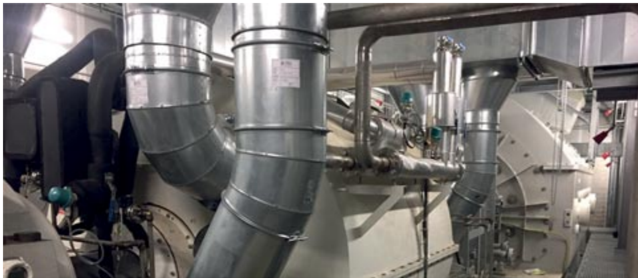
Figure 10 – Site photos - Flywheel and Synchronous Condenser inside the weatherproof enclosure
